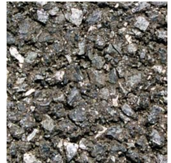
Close-up of the road surface defined by the directive
