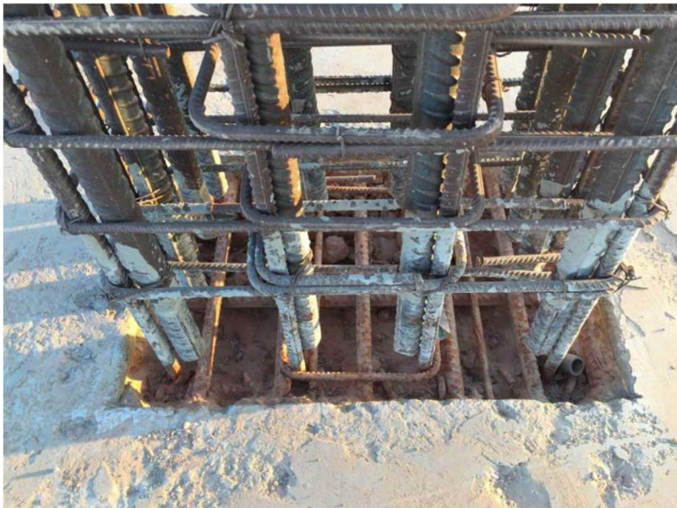
Wrong anchoring of P2 starter bars
